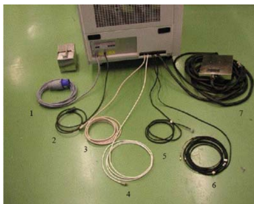
Figure 10.16 External Imaging Rack Cables
